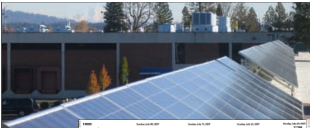
Solar panels on top of Vernier roof with a view of Mt. Hood in the background
