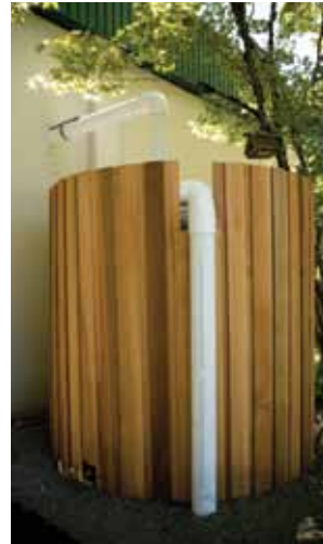
Rainwater capture tank provides water for lawn
